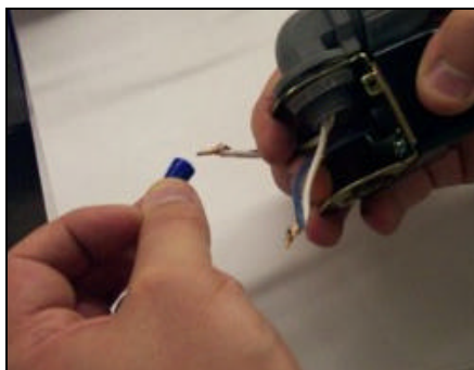
Removing the wire nuts
