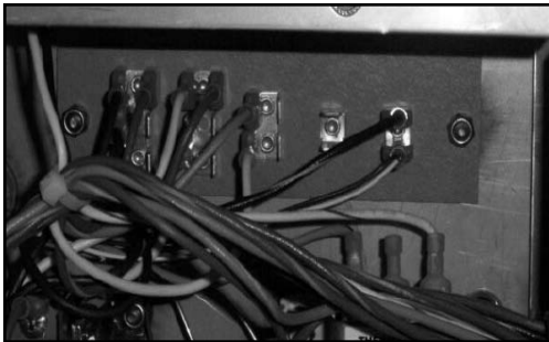
Terminal board inside the heater box
